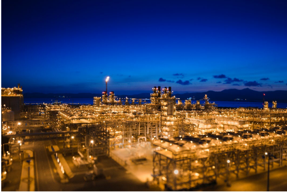
LNG (liquified natural gas) plant on Curtis Island. Image courtesy of Shell's QGC business
